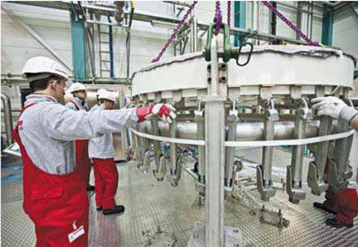
Building a turnkey factory: employees of Centrotherm install a so-called CVD-reactor for silicon production. (Source: Centrotherm)
