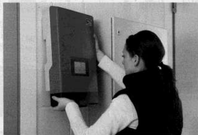
Foto: SMA Solar Technology AG
