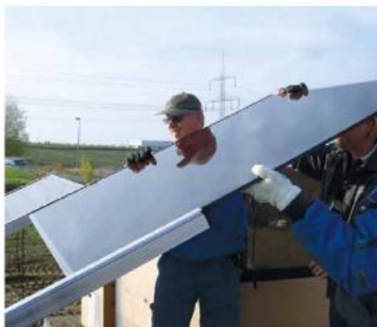
Fast enough? Even solar technology engineers can reduce costs – by providing more efficiency for rooftop installations in the shortest time. (Photo: Bosch)
