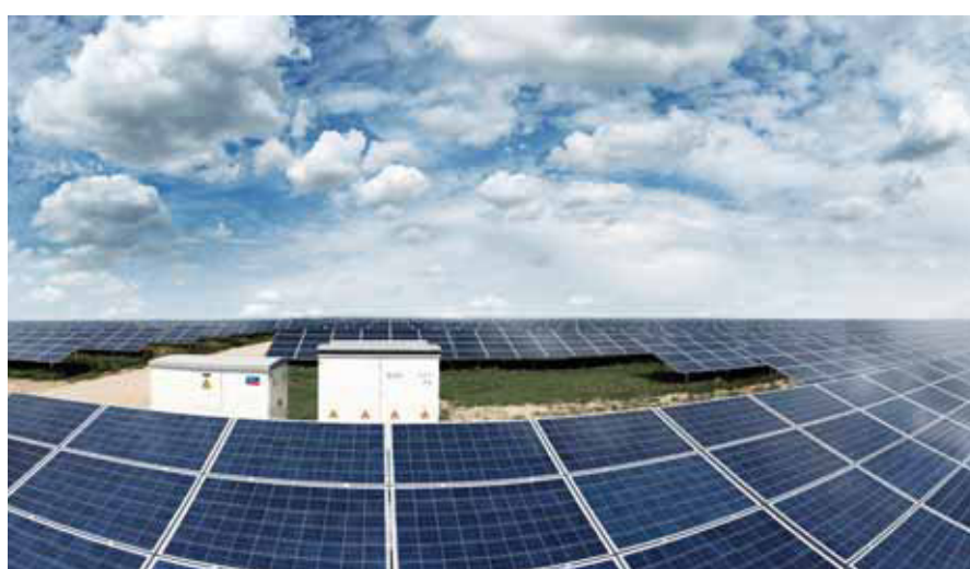
Right: Too much solar power? Solar power necessarily involves fluctuations. Batteries are therefore required to make it predictable (photo: SMA).
